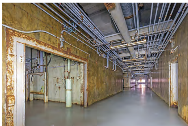
RSL 1 RLOB frozen spine corridor looking towards open entrance doors. Photo Chris Howells
